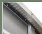
Tank Gutter System
